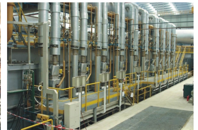
步进加热炉驱动 Step Heating Furnace Drive
